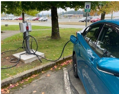
Port Alberni Campus EV Charging Stations
