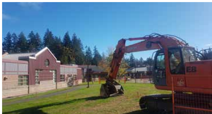
Construction crews break ground on the new Indigenous Gathering Place at NIC's Campbell River campus.
